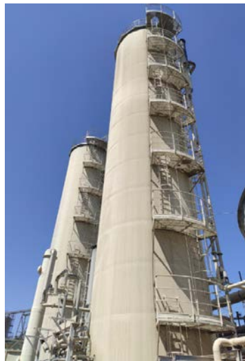
Figure 19. Biogas digester in WWTP.
